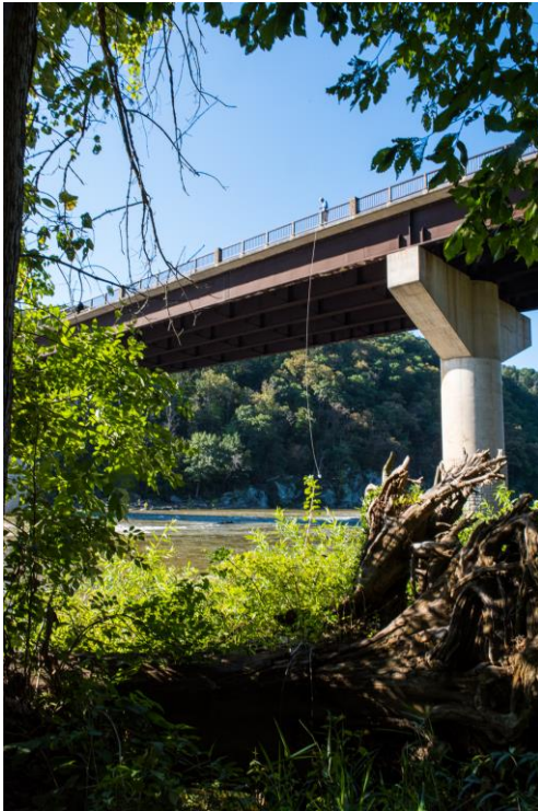
Figure 2. Rt. 340 bridge over Shenandoah River near Harpers Ferry, WV (R. Bourassa, ICPRB).
