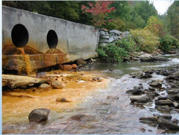
Acid mine drainage, McDonald Mine, 2012. Photo by ICPRB.
