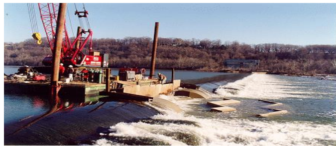
Construction of the Little Falls Fishway. Photo Courtesy of the U.S. Army Corps of Engineers.
